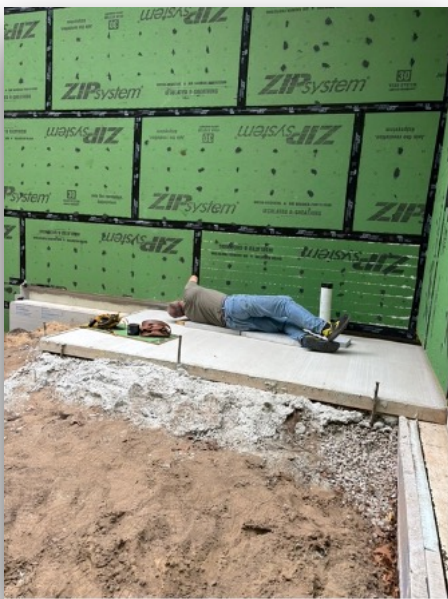
Zip-R Sheathing: tape joints, caulk nail heads, & apply Siga Fentrim 430 (grey tape) to seal concrete & mud sill interface.
